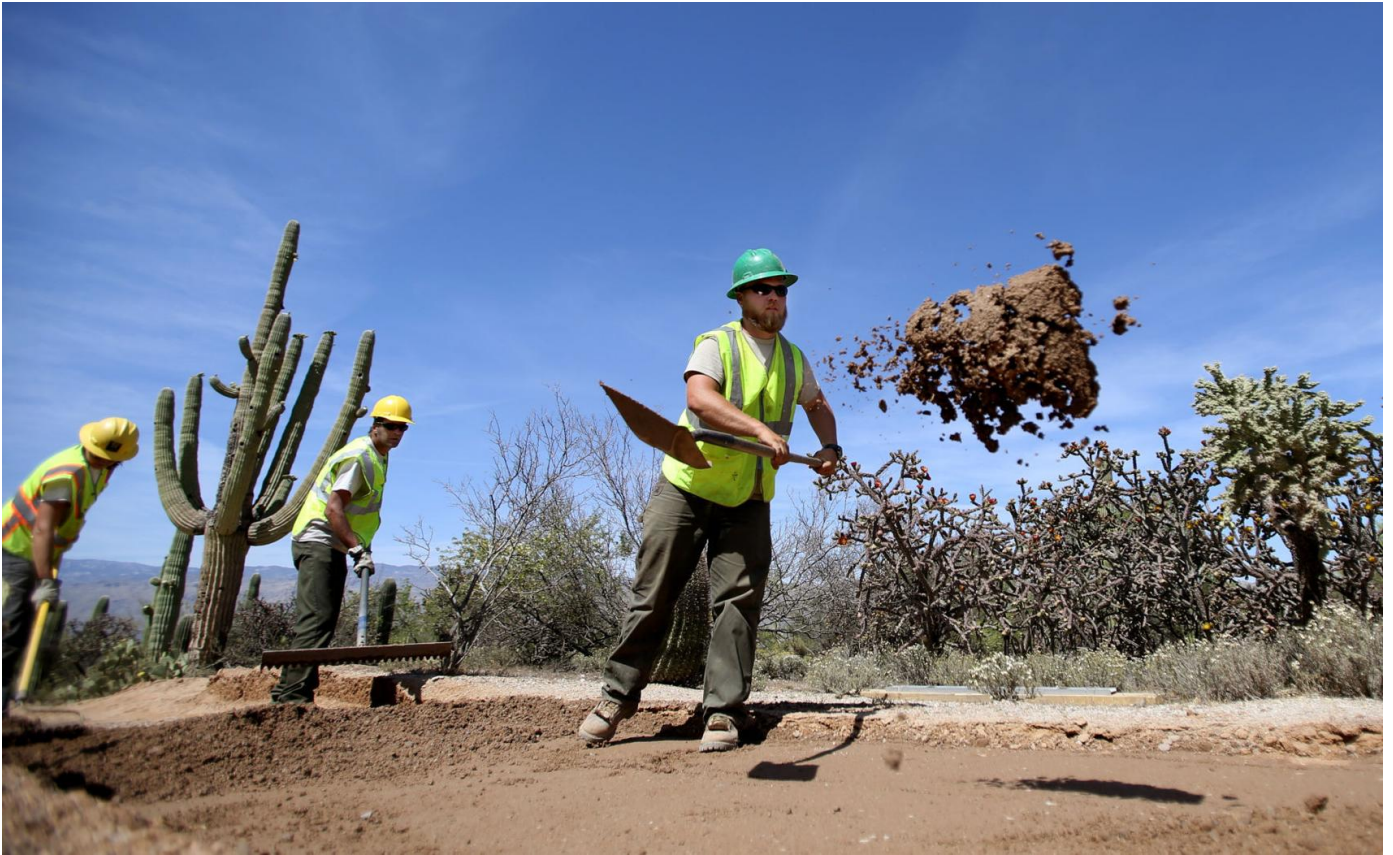
Trail worker Brad Duffe redistributes material as he and his trail crew lay down a bed for a new surface, part of remodeling the Mica Springs Trail to make it ADA compliant in Saguaro National Park East on April 22, 2016.
